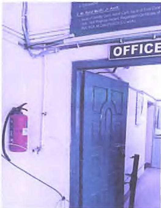
Fig. 8: Fire Extinguisher fixed in front of the office
